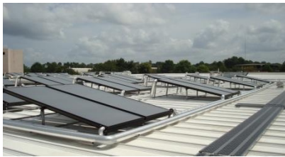
Solar panels at Jail North facility.
